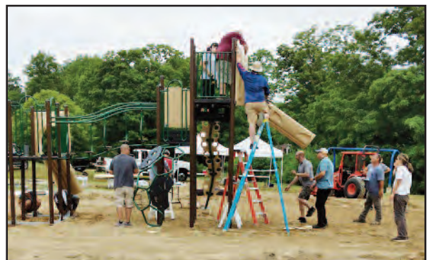
Managed as a “community build project” the new playground was installed with oversight by the contractor with the School Principal leading parents and volunteers.
